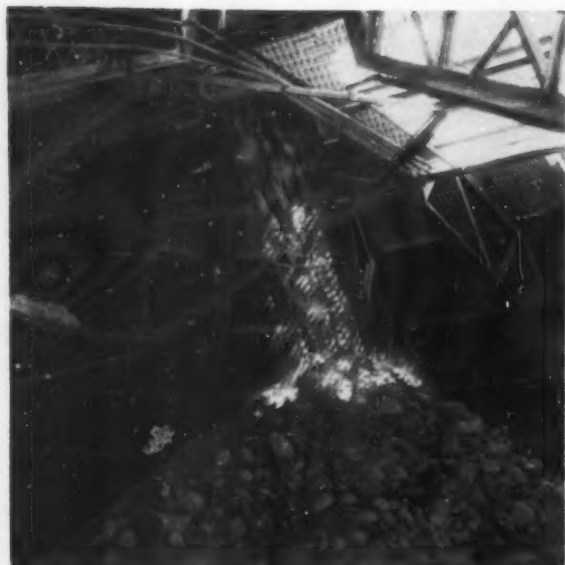
TELEVISION camera view of covered coarse ore storage bin at end of 975 foot long belt conveyor.
